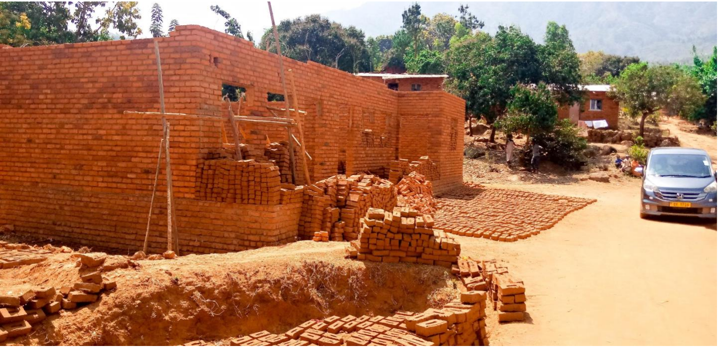
The above picture shows Malakamu school construction which was temporarily stopped the past two weeks. The villagers have now started moulding additional bricks at the construction site for convenience, which will be burnt for the completion of the school structure, a kitchen and a bakery and toilet.
