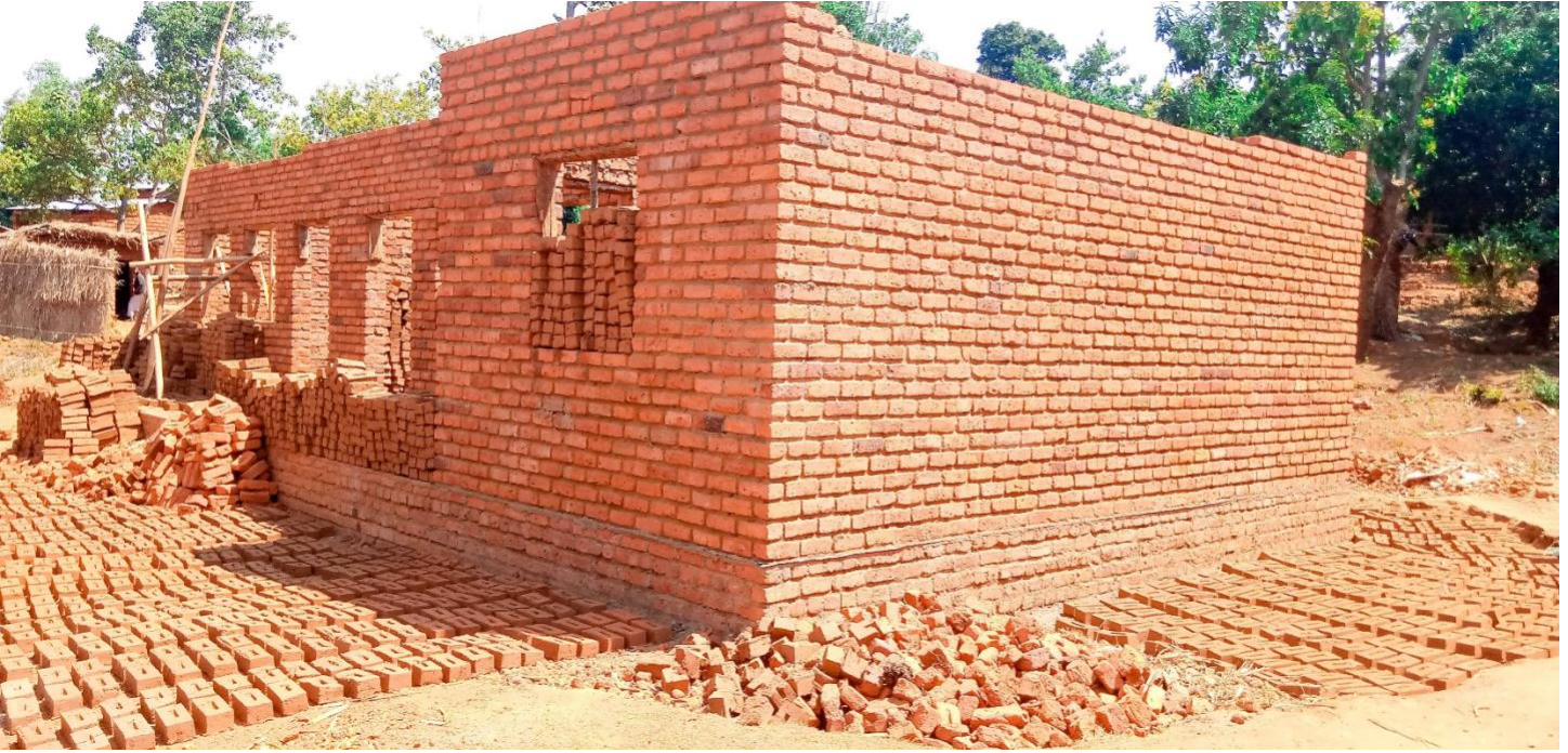
Left front angle view of the building. New bricks are laid around the building waiting to be burnt by the community.
